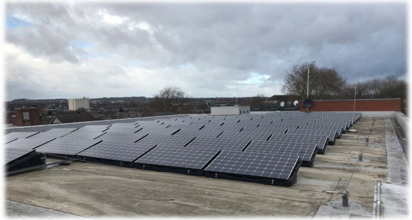
Solar panels on roof of new development, Nottingham
