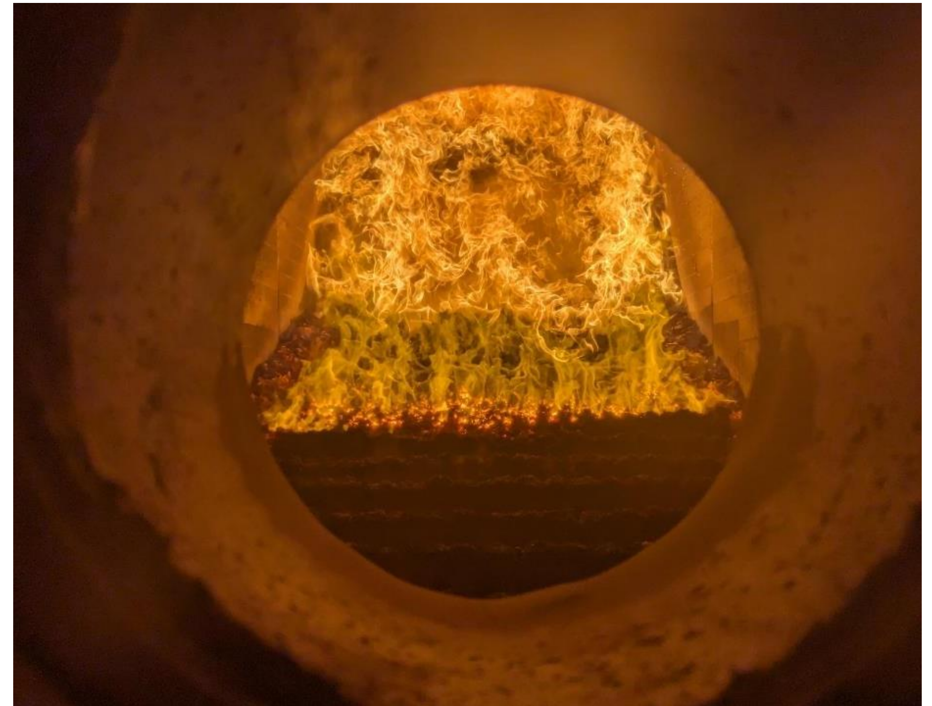
Combustion chamber, 1MW biomass steam boiler, Nc'nean Distillery
